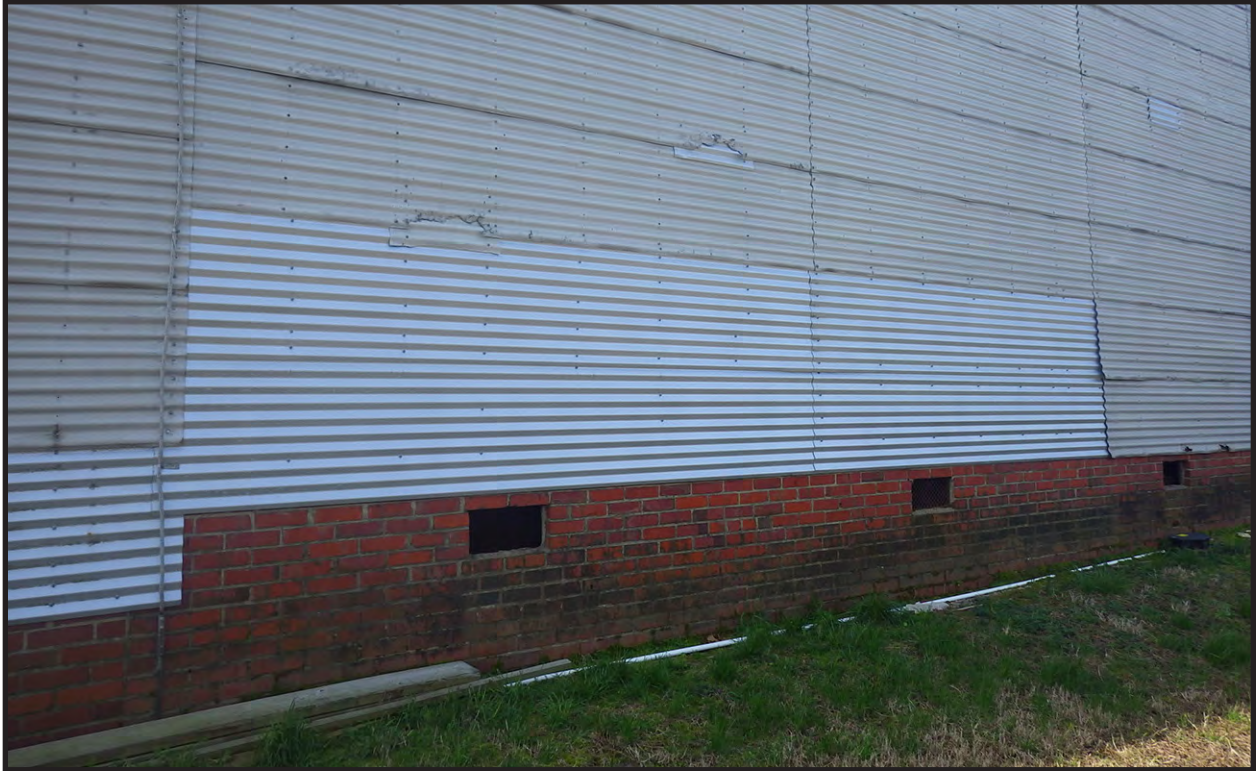
Figure 9. North Side of Main Complex Showing Original and Replacement Siding
